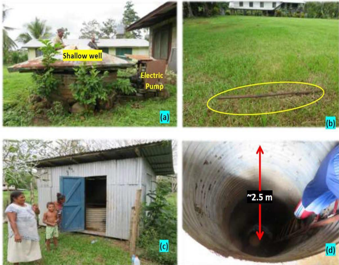
Figure 3: Water supply system at Kubuna. (a) Shallow well near priest's residence. (b) Remains of 20 mm water supply pipe (yellow circle) from the spring located 500 m west. (c & d) Shallow well near the Pastoral Centre building.
